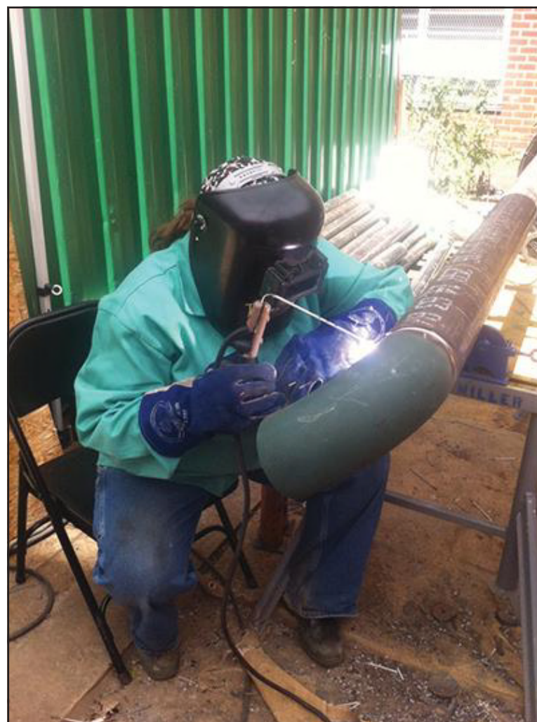
Powers welding at the Penn Station South complex, which Local 638 help modernize.
