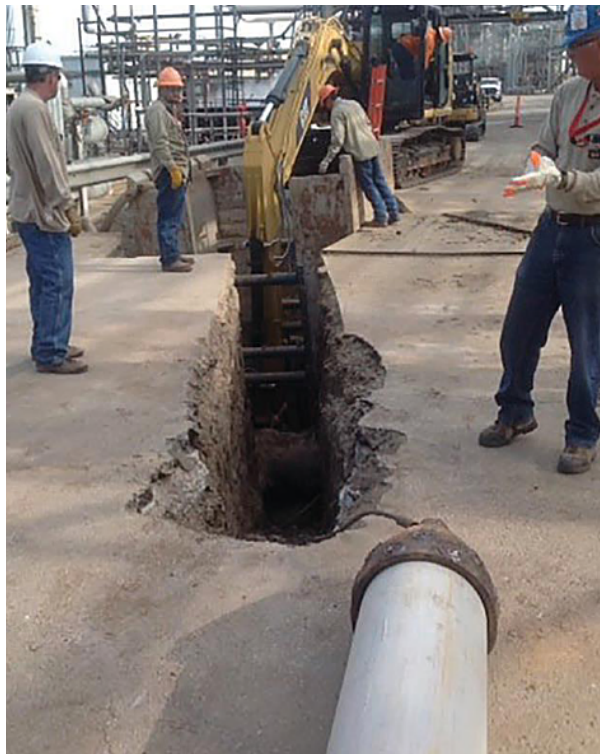
Below: Midpoint access pit excavation on existing sewer main that crossed under refinery fire protection system pond and under active refinery units.
