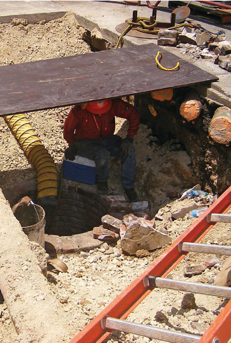
Below: Preparation for a 12-inch HDPE pipe-bursting pull under an existing refinery process unit.
