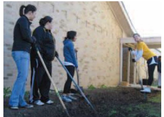
(Above) Members of Kappa Pi Gamma help prepare the foundation for a brick path to the Mosaic Community Garden during the Day of the Dogs in February.
